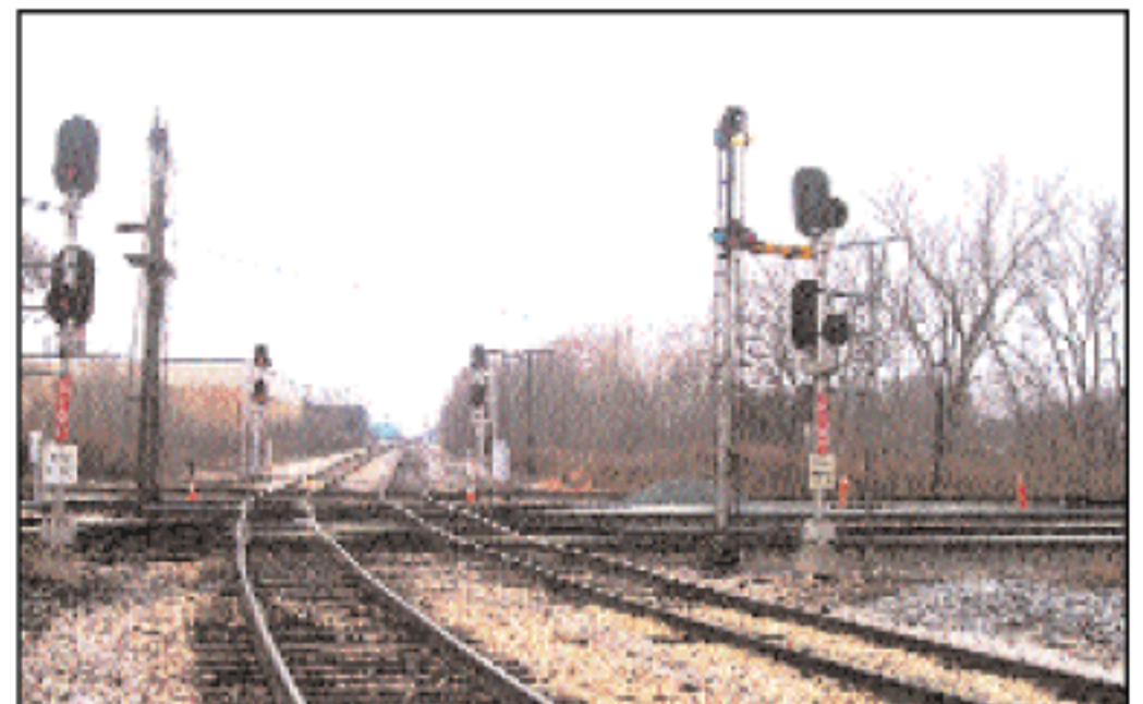
Typical Signal Installation
