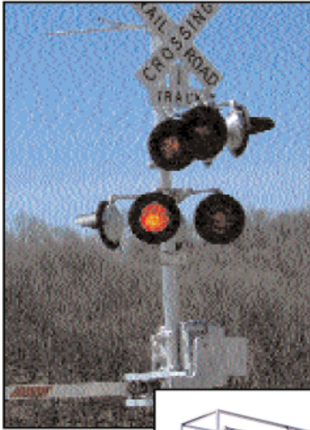
Flashing Lights and Gate Mechanism
