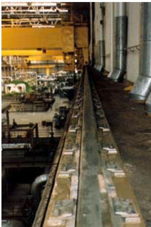
Nuclear Power Station Tricastin (F) - Weldable clips
